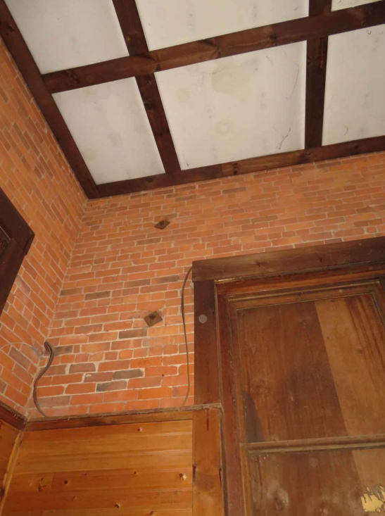
BRICK DAMAGED BY BRACKET FASTENERS
