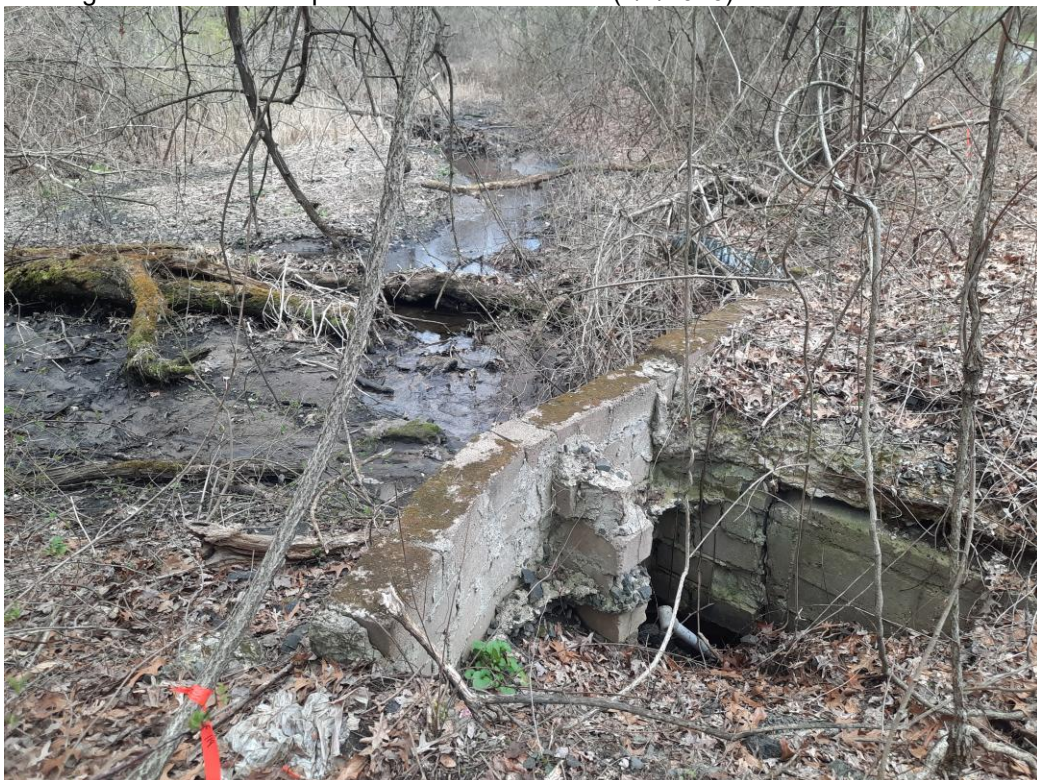
Compromised outlet structure. Note former pond in background (4/7/2026).
