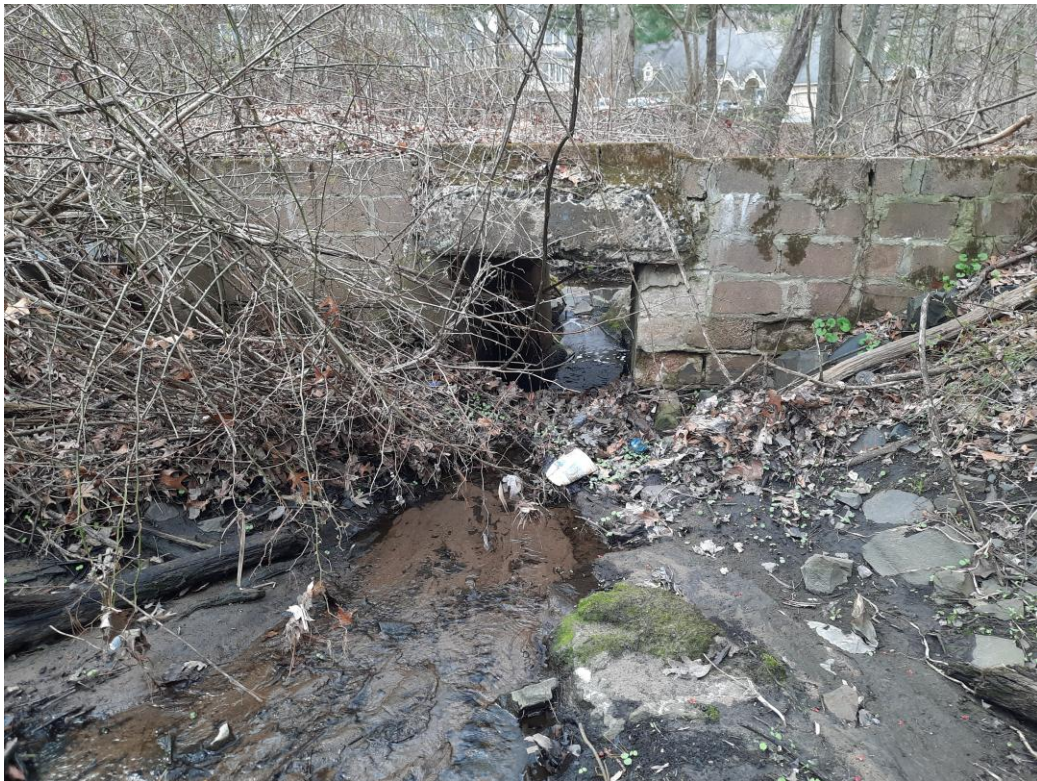
Looking southwest at compromised outlet structure (4/7/2026).
