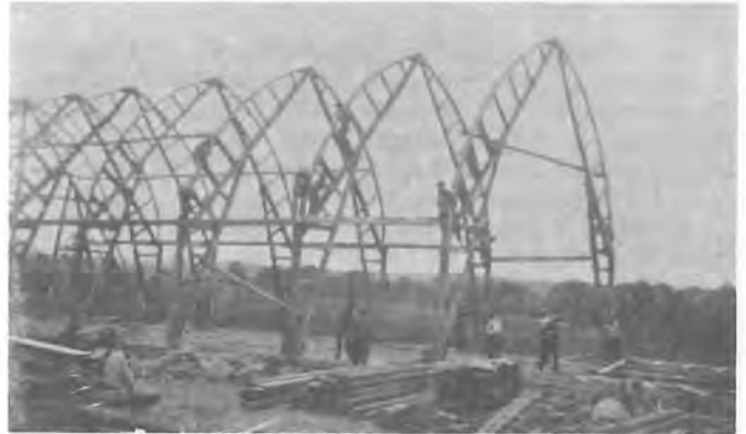
Barn raising on the Sigmund Woller farm after a fire that destroyed the barn in 1947. This design is typical of the newer structures called hip roofed barns.
