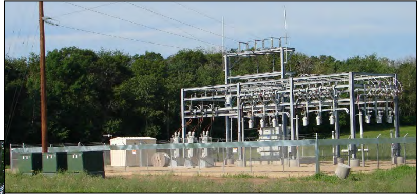
Photo: The Boardman electrical substation is one of several utility facilities located in the Town of Richmond.
