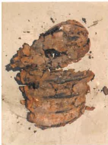
FAILED CORRUGATED METAL PIPES TO BE REMOVED AND REPLACED AS NEEDED
