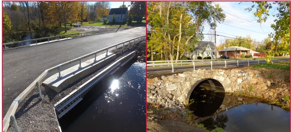
Rathburn Road Bridge, Town of Oswego Walmore Road Culvert, Town of Wheatfield
