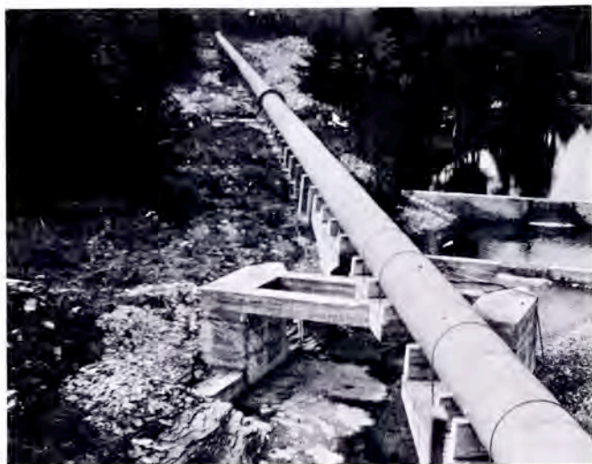
The penstock from the McGregor dam to the McGregor power house showing the support where it crosses the river.
