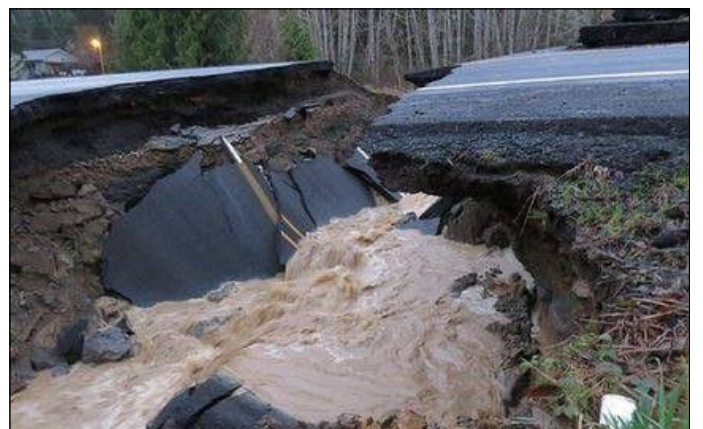
Heavy Rain A collapsed culvert on SR 4 near Nassel in January 2015. PCEMA Photo.
