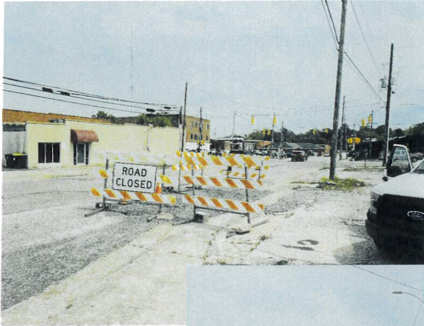
Latest King Street Surface Failure -- 52' x 10' Area
