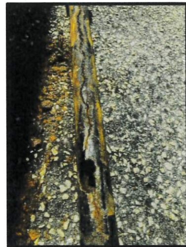
Rusted Drain Line From Lab
