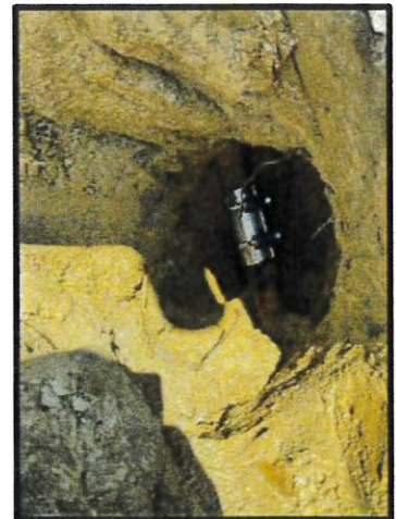
Figure 4 - 2" Water Leak Repair
